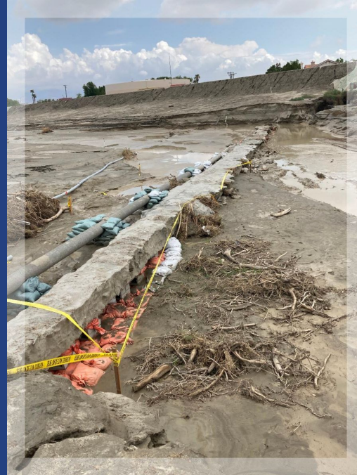
Looking east, showing Indio Water Authority's (IWA'S) steel reservoir at the top of the embankment. Next to our concrete-encased sewer main (rectangular structure) is IWA's water pipeline, also exposed during the initial storm of February 14, 2019.
