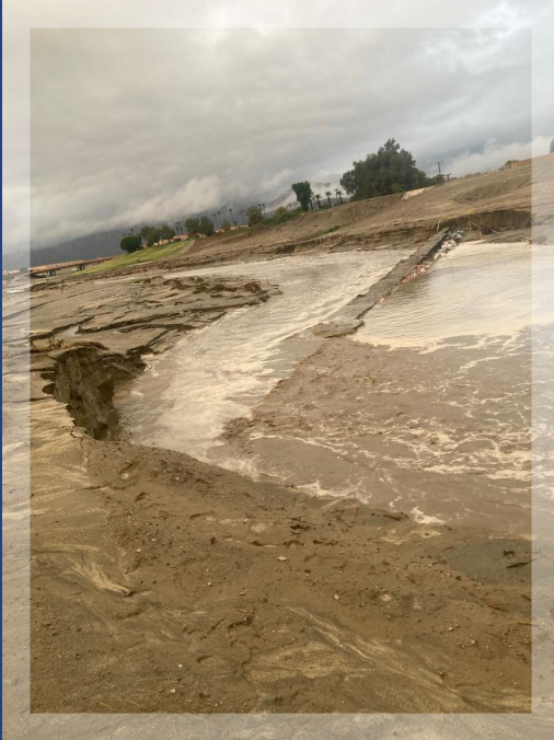
Looking west, with Westward Ho Drive in Indio at the top of the embankment, showing the channel filled with water after a storm event.
