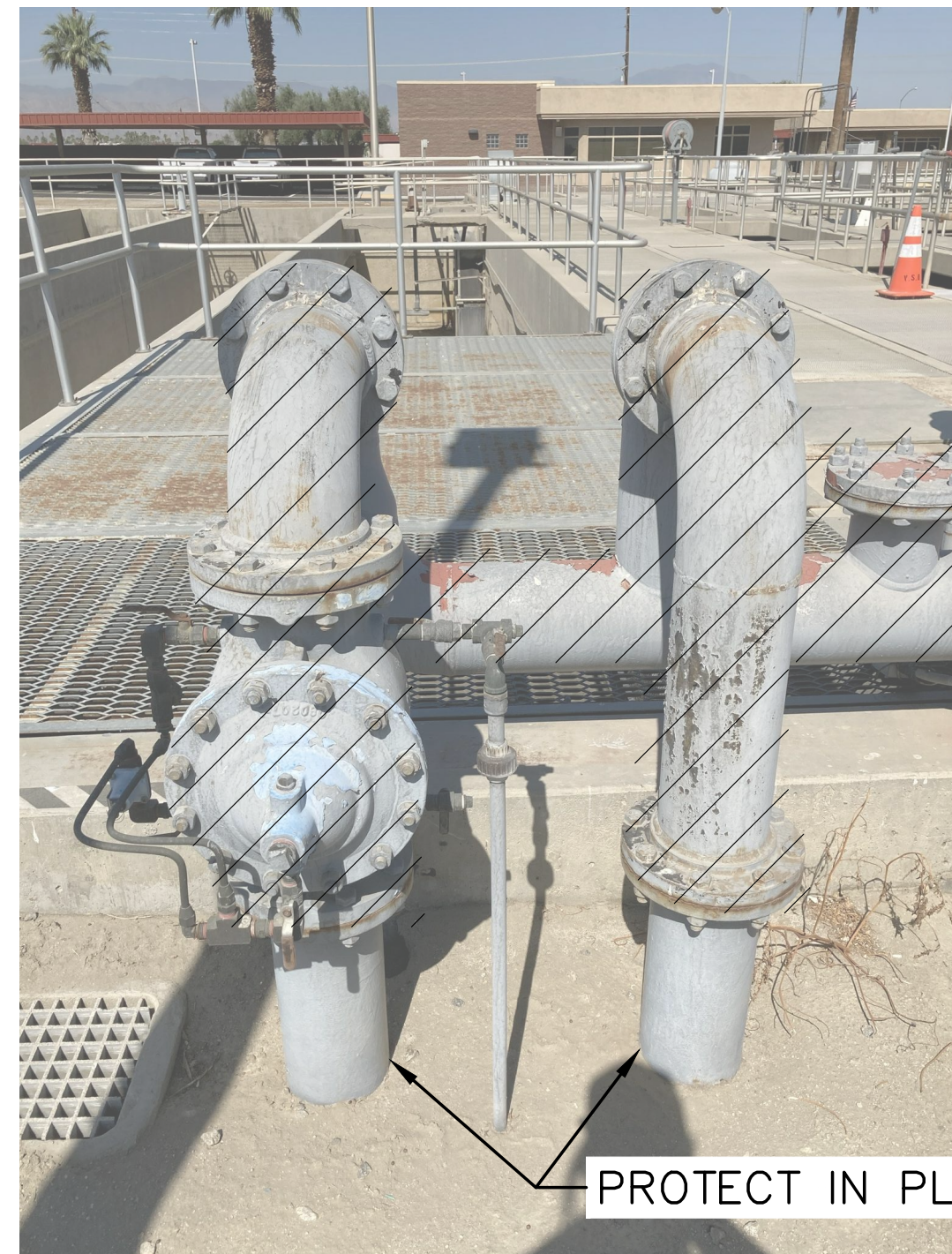
PHOTO EXISTING PIPING TO BE DEMOLISHED (G)
