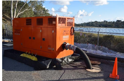
Bypass pumping setup as part of a headworks rehabilitation project at the San Elijo WRF.
