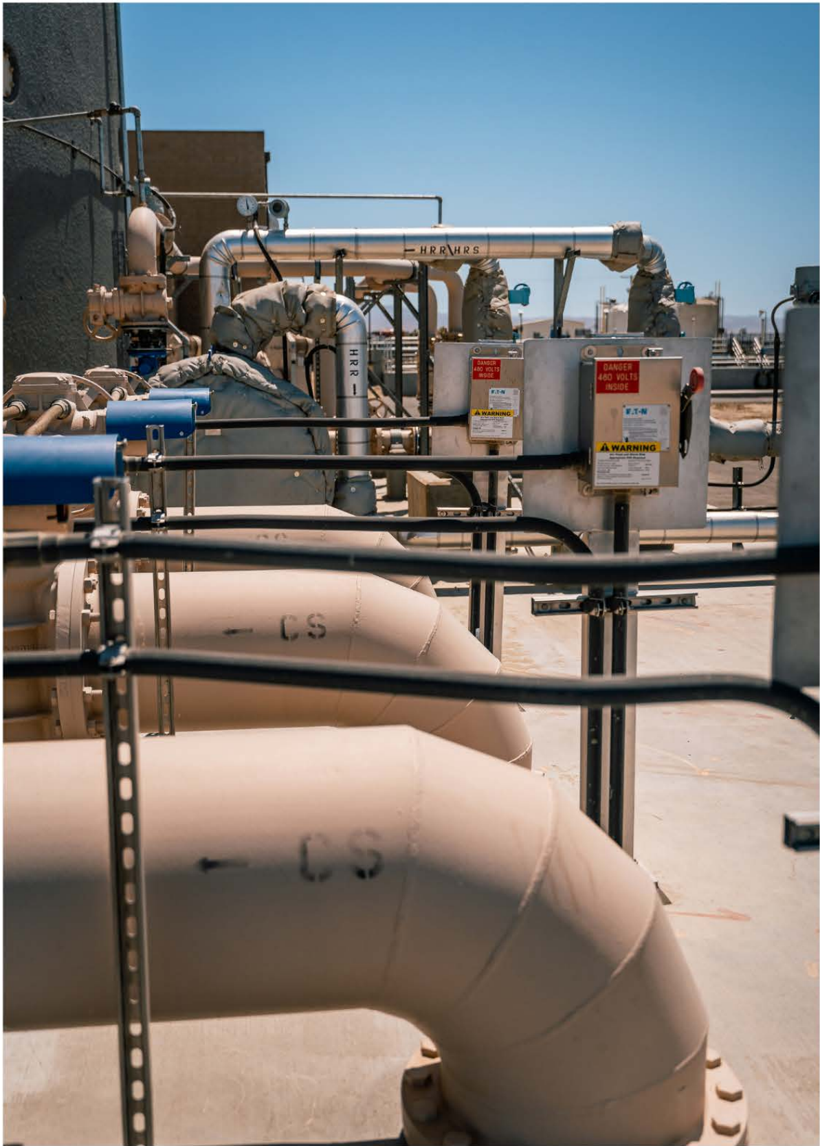
Digester Heating Pipes
