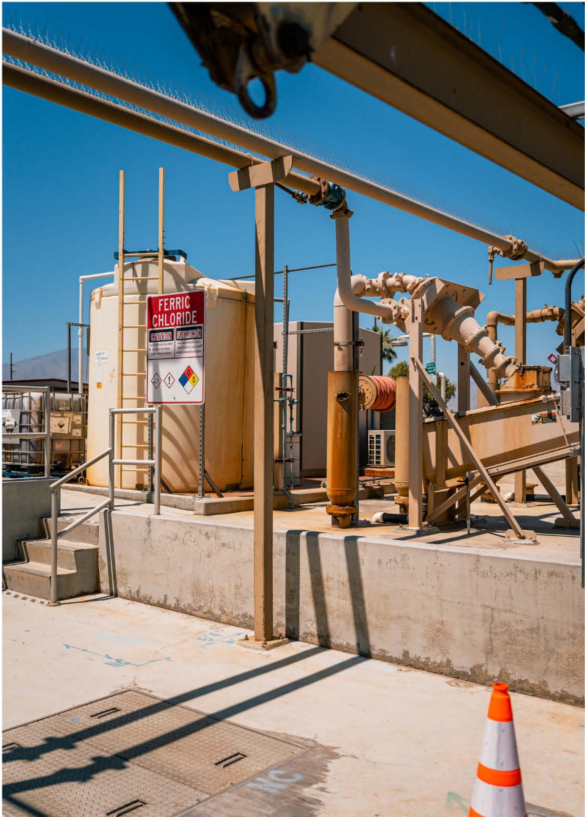
Ferric Chloride Tank
