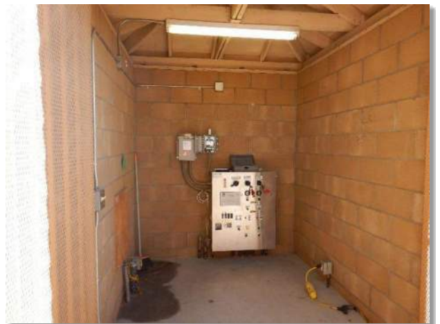
Photo 3-28. Electrical building interior
