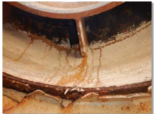
Photo 3-56. Moderate corrosion on framing where coating has delaminated
