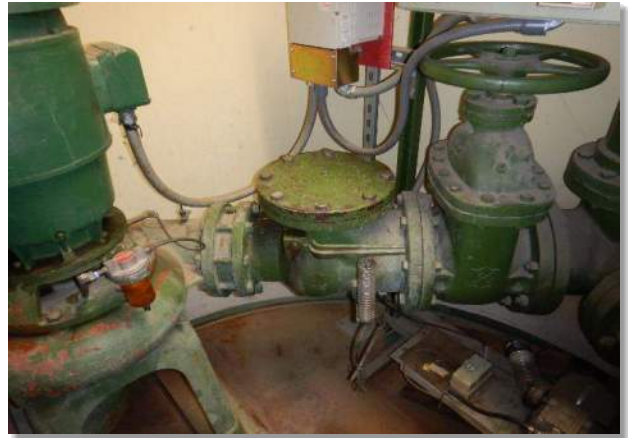
Photo 3-12. Pump No. 2, discharge piping and valves
