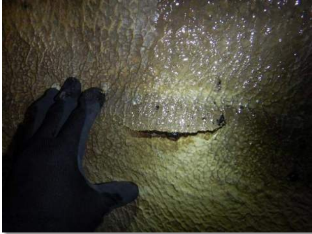
Photo 3-37. Tearing in liner, typical throughout
