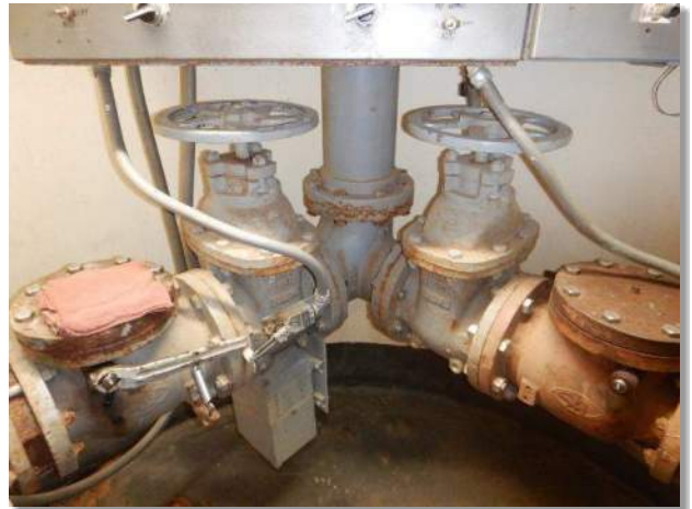
Photo 3-66. Discharge piping and header
