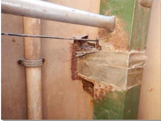
Photo 3-57. Moderate corrosion at ladder entry system interface with wall
