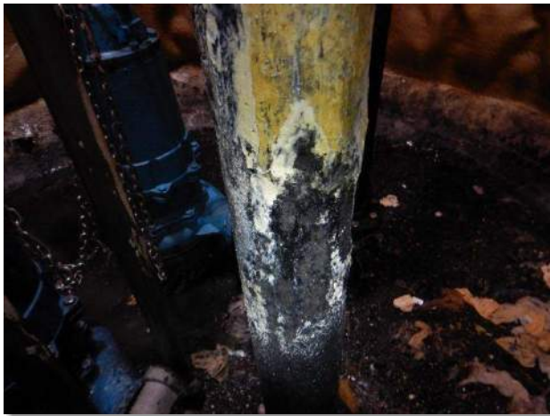
Photo 3-45. Moderate corrosion between 5-ft to 6-ft level of the wet well, typical both discharge pipes
