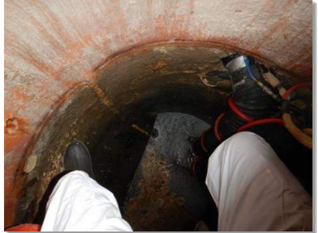
Photo 3-74. Wet well interior, liner degraded below waterline
