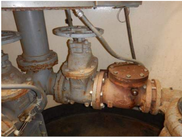
Photo 3-65. Pump No. 2 discharge piping and valves
