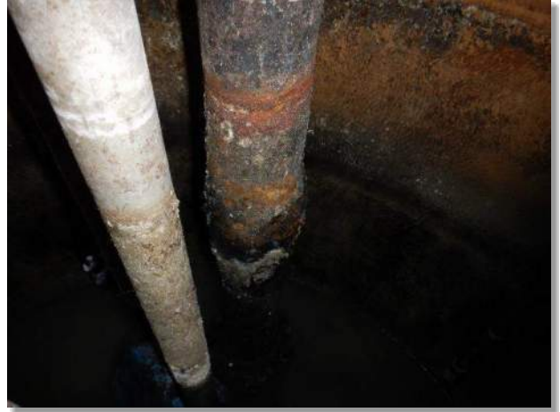
Photo 3-92. Severe corrosion at Pump 2 discharge piping
