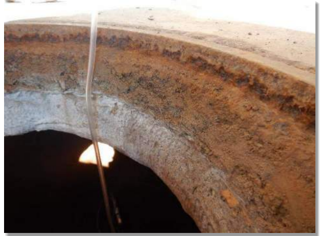
Photo 3-16. Severe corrosion & metal loss at the rim
