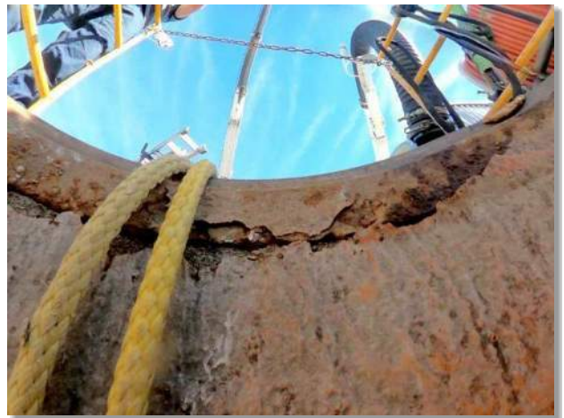
Photo 3-72. Moderate corrosion at rim where lining has deteriorated
