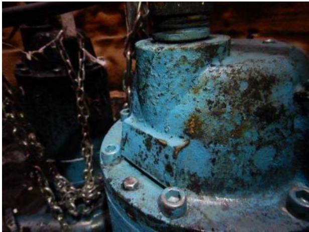
Photo 3-51. Minor surface corrosion at Pump 2
