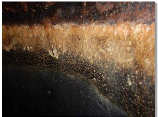
Photo 3-20. Blistering in liner (approximately 2-in) around circumference near lower termination point
