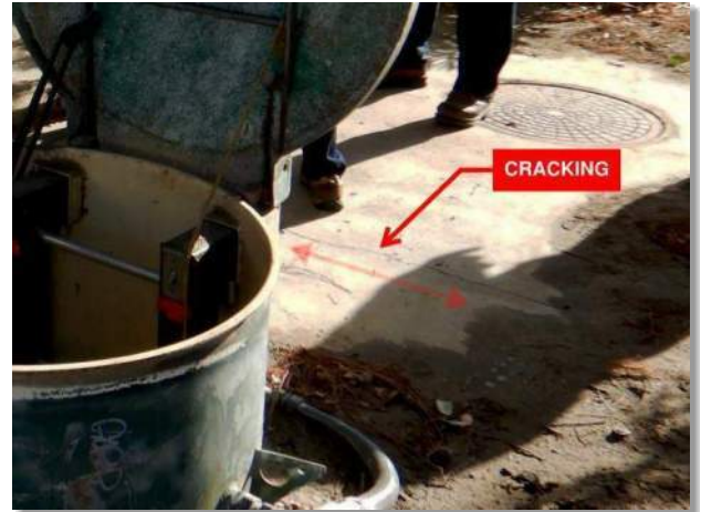
Photo 3-2. Cracking on exterior slab, facing east
