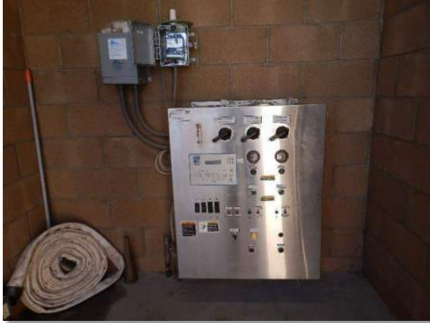
Photo 3-29. Lift station control panel
