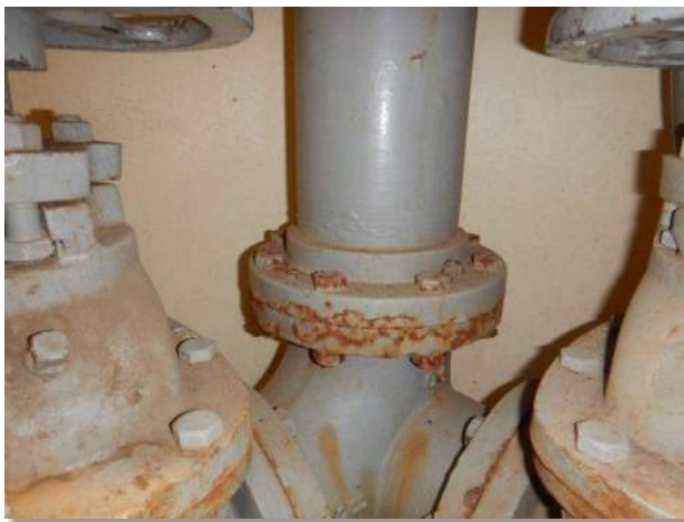
Photo 3-67. Discharge header, minor corrosion at flange
