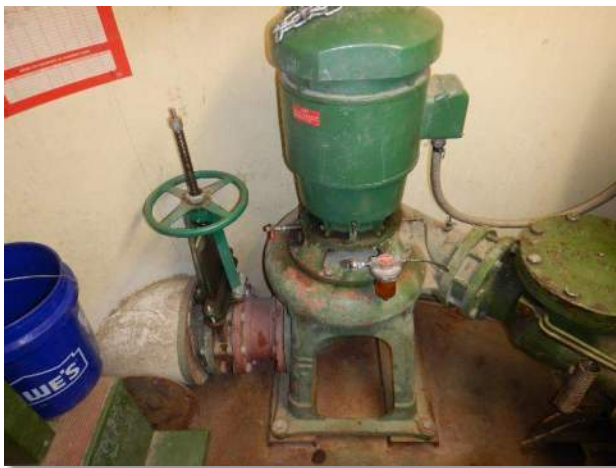
Photo 3-9. Pump No. 1, suction piping and valves
