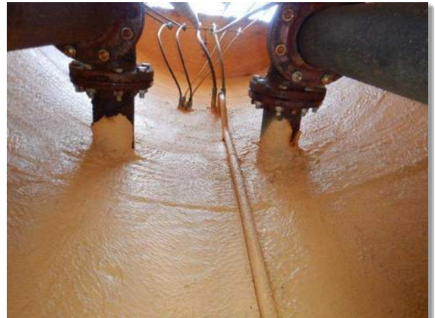
Photo 3-88. Pump discharge piping wall penetration, wet well interior lining in good condition.
