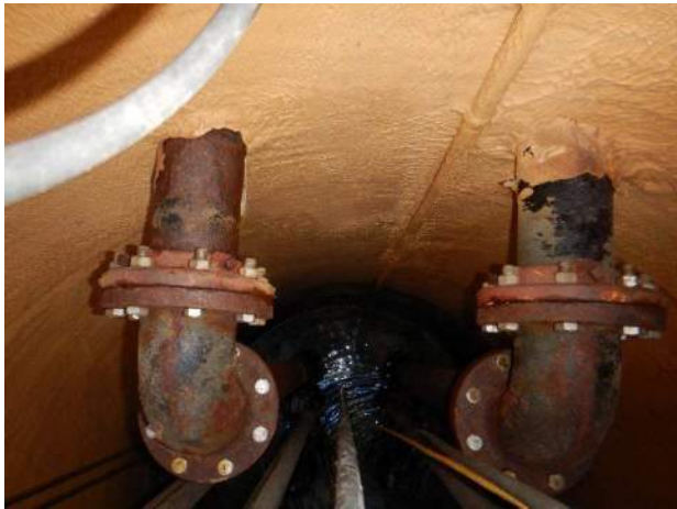
Photo 3-87. Moderate corrosion at elevated pump discharge piping
