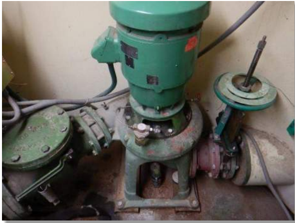
Photo 3-11. Pump No. 2, suction piping and valves
