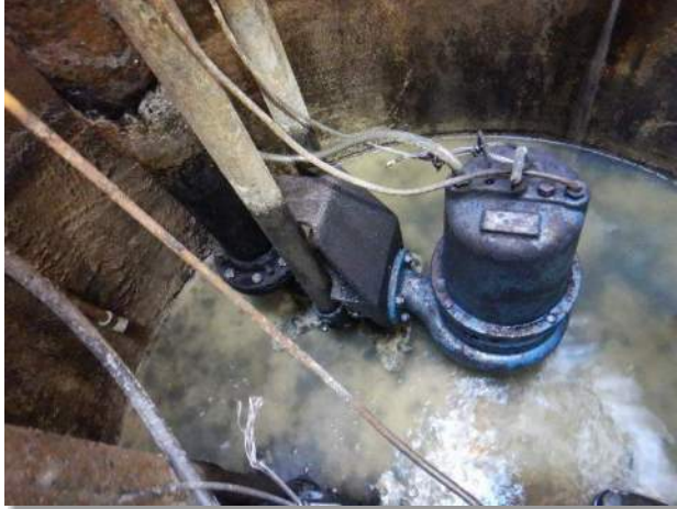
Photo 3-85. Pump No. 1 (south)
