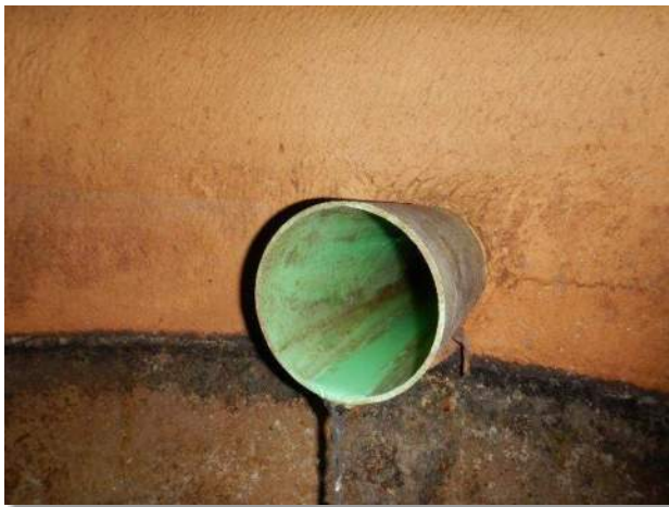
Photo 3-83. 6-in PVC inlet pipe
