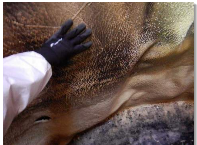
Photo 3-36. Severe delamination, closeup at lower section of wet well
