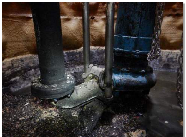
Photo 3-48. Pump 1 discharge piping
