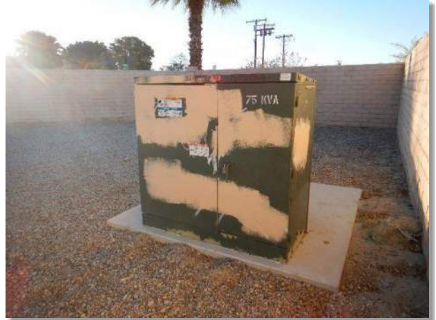
Photo 3-30. Coating deterioration at pad-mounted transformer
