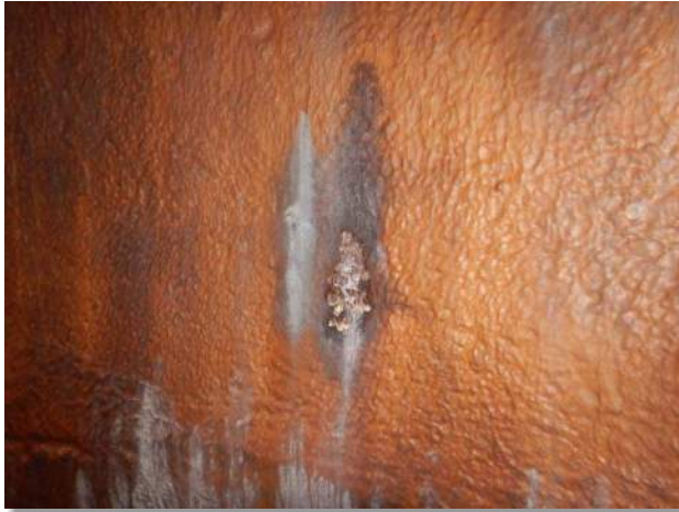
Photo 3-21. Blistering in liner, typical of 2 locations approximately 4-ft below the rim
