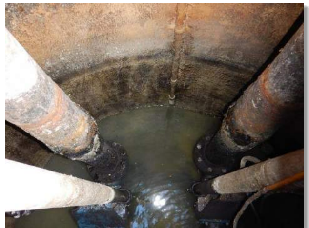
Photo 3-90. Severe corrosion of DIP discharge piping at operating level
