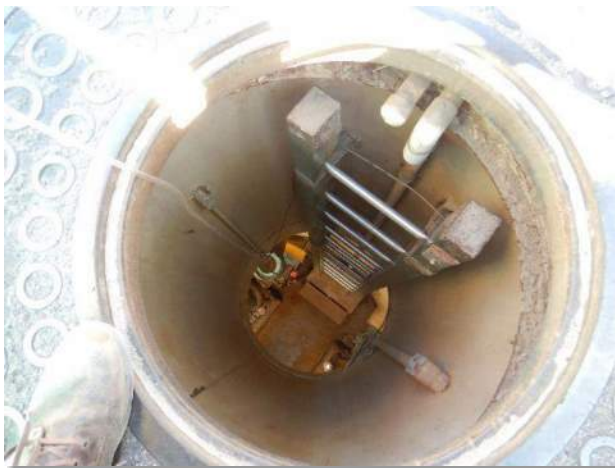
Photo 3-55. Dry well topside, minor offset in framing
