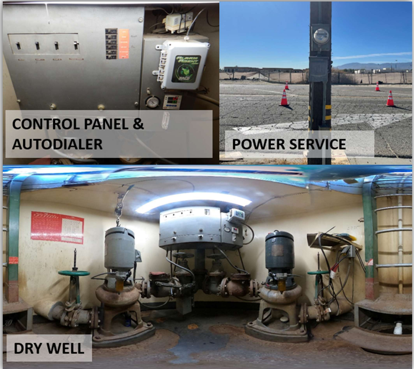
FIGURE 7: Carver Lift Station Photos
