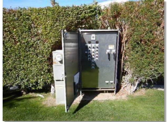
Photo 3-78. Pump control panel
