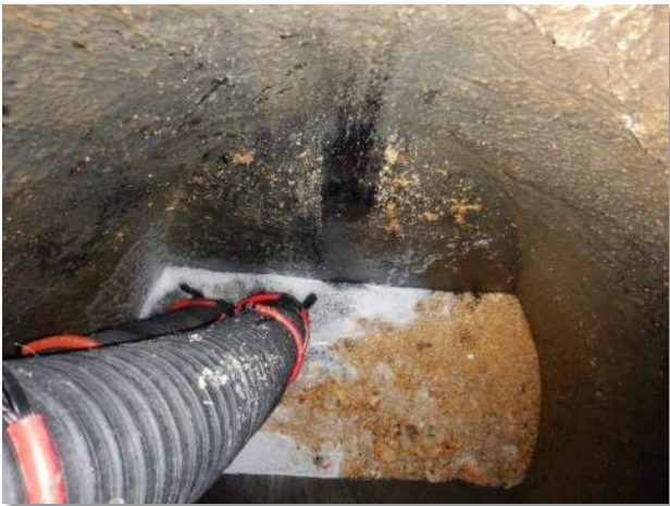
Photo 3-75. Wet well sloped walls, channel
