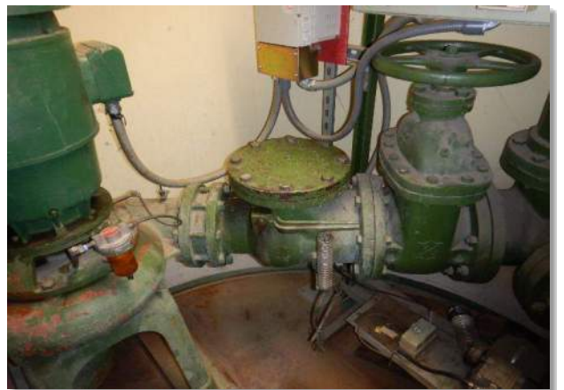
Photo 3-10. Pump No. 1, discharge piping and valves
