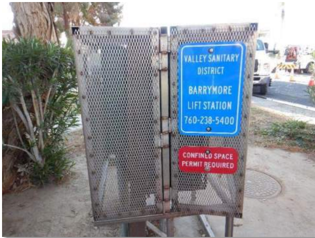
Photo 3-3. Barrymore LS control panel
