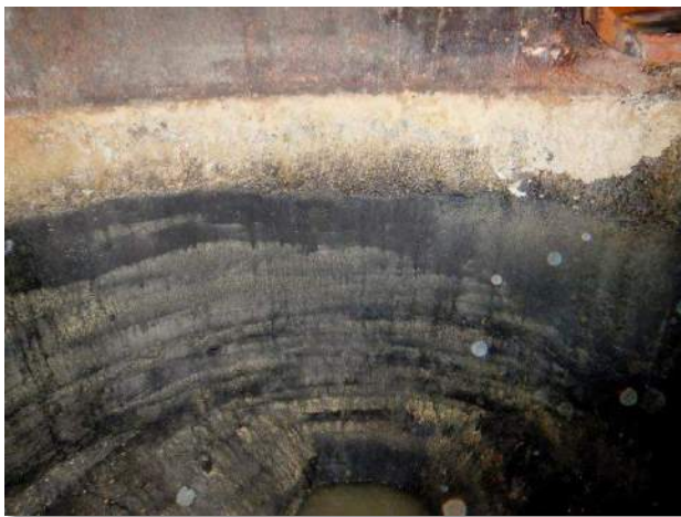
Photo 3-19. Lower 4-ft of wet well unlined
