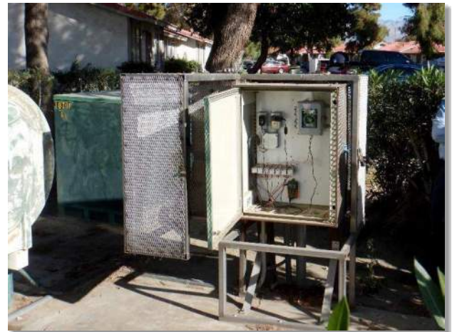
Photo 3-4. Barrymore LS control panel (open)
