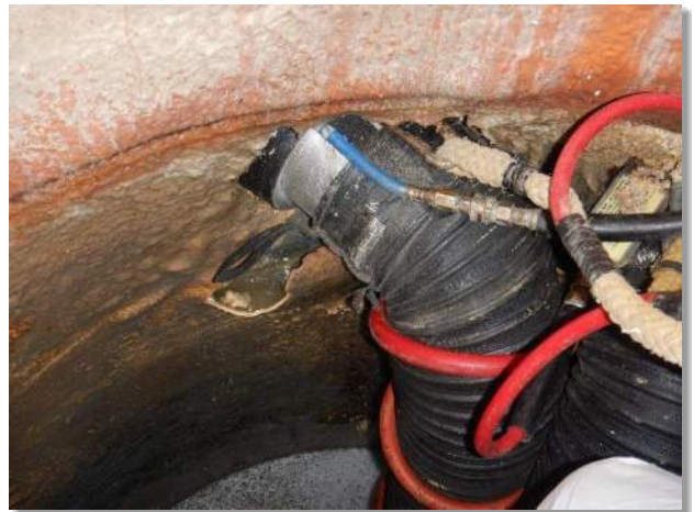
Photo 3-76. Liner torn and retaining water beneath drop-in laterals
