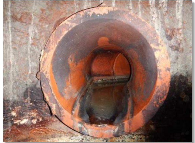
Photo 3-22. Wet well influent pipe
