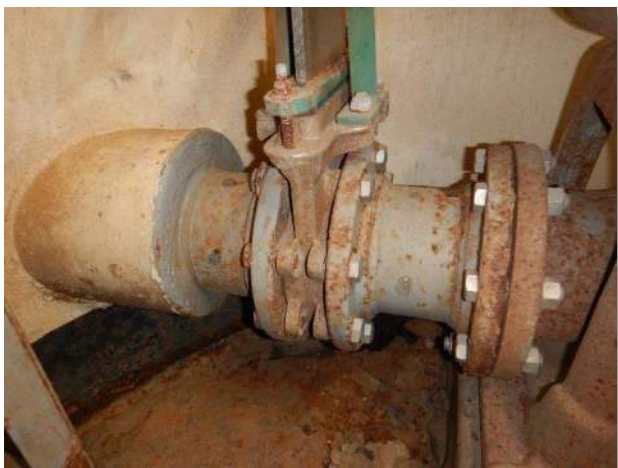
Photo 3-61. Pump No. 1 suction piping & valve
