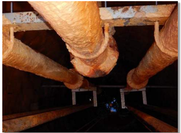
Photo 3-46. Corrosion staining evident throughout discharge piping
