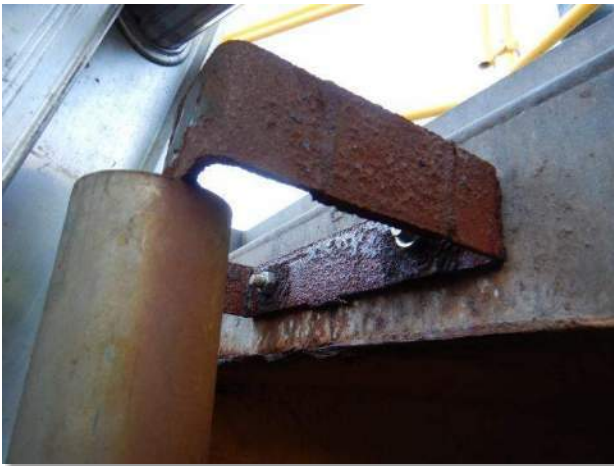
Photo 3-93. Moderate corrosion at mild steel supports
