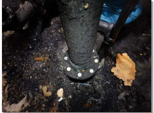
Photo 3-50. Pump 2 discharge piping
