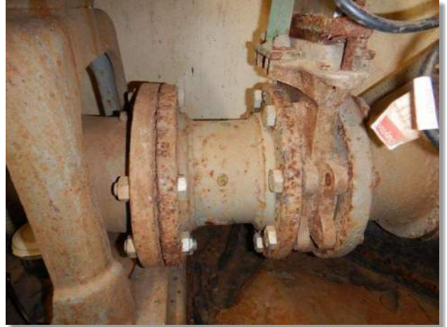
Photo 3-64. Pump No. 2 suction piping & valve
