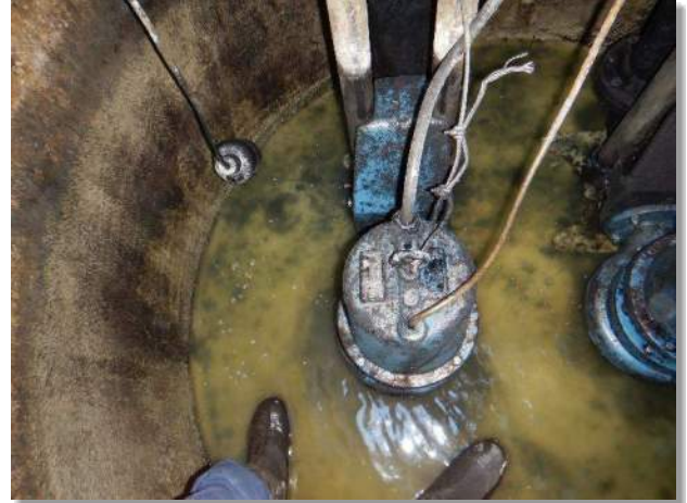
Photo 3-86. Pump No. 2 (north)
