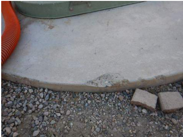
Photo 3-33. Minor spalling on exterior concrete pad, likely due to impact damage
