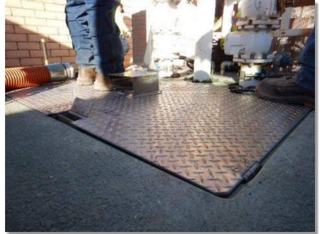
Photo 3-32. SST access hatch
