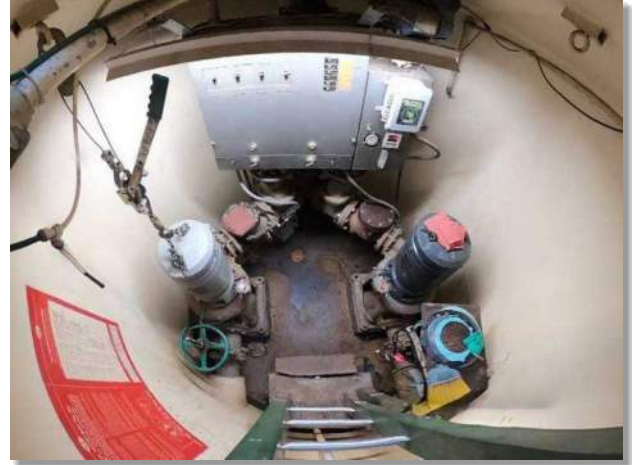
Photo 3-58. Dry well interior, 360 view (cropped)
