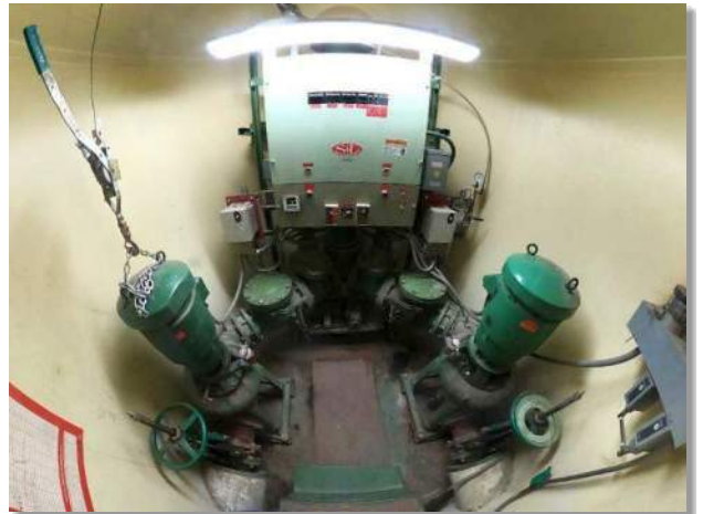
Photo 3-8. Dry well interior, 360 view (cropped)
