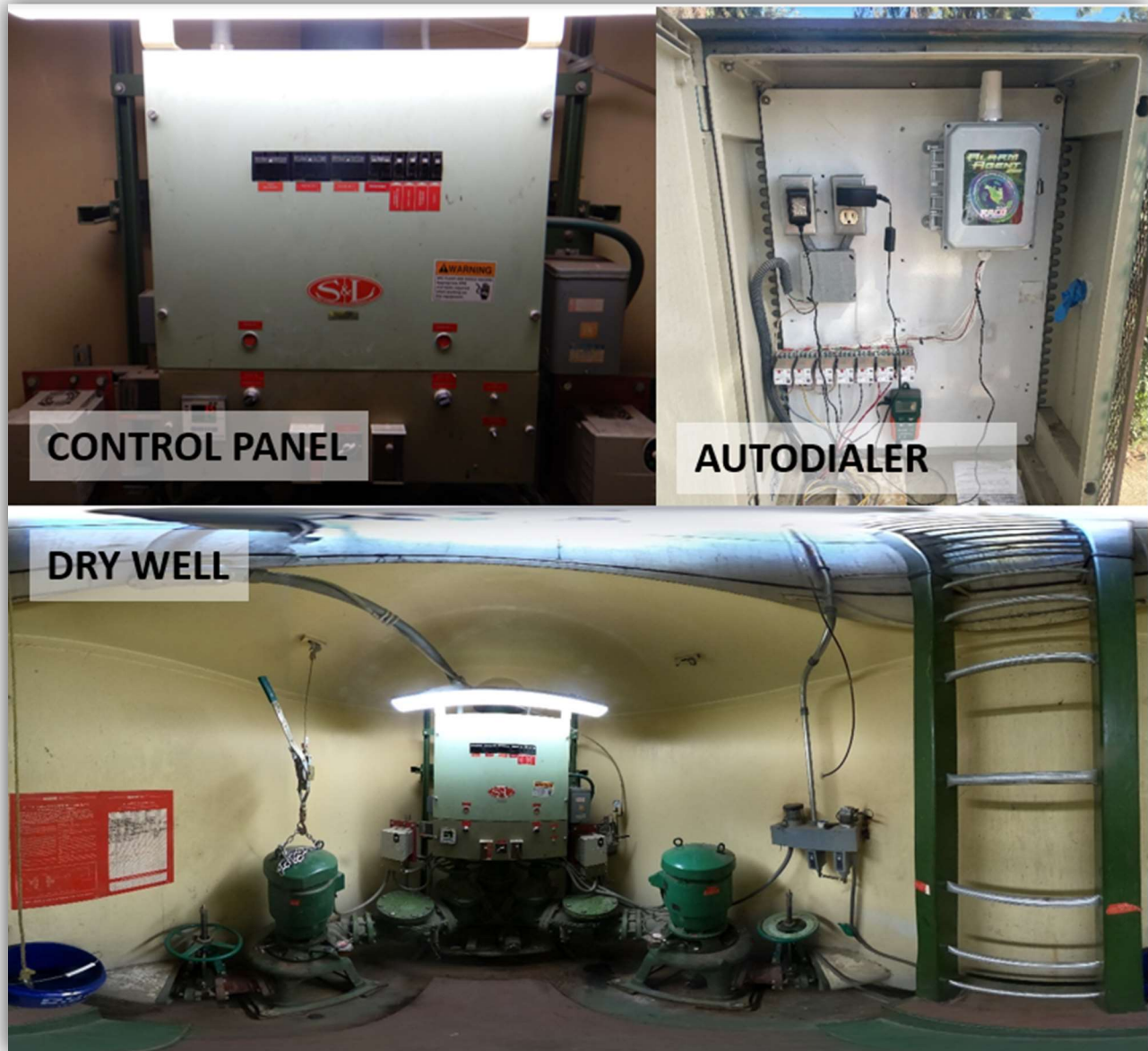
FIGURE 5: Barrymore Lift Station Photos
