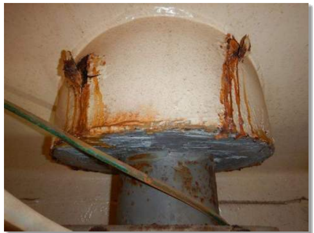
Photo 3-68. Discharge header, minor corrosion at ceiling penetration
