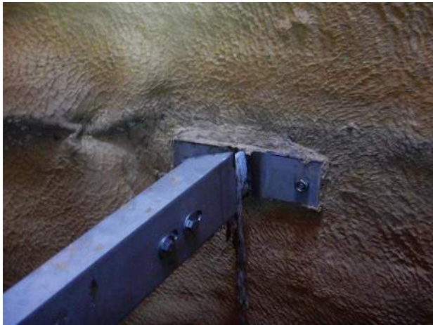
Photo 3-39. SST guide rail supports & hardware
