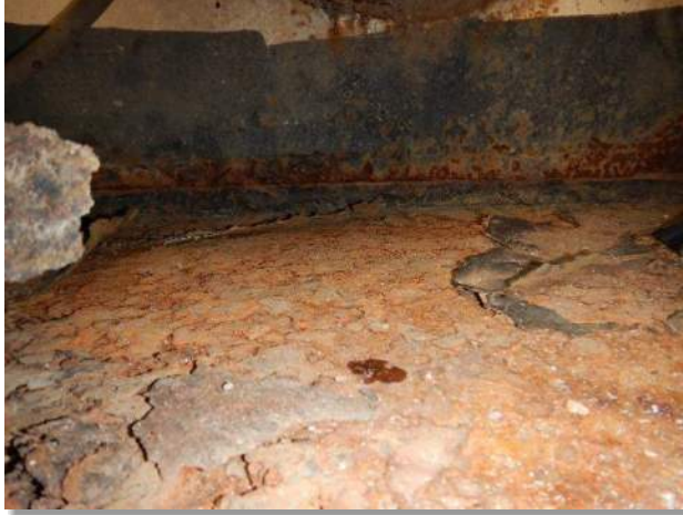
Photo 3-69. Moderate corrosion at floor plate
