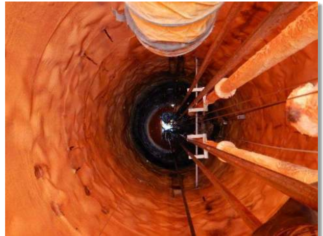
Photo 3-34. Wet well interior, topside
