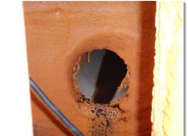
Photo 3-40. Emergency PVC overflow
