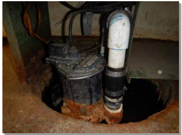
Photo 3-14. Moderate corrosion below waterline in sump area & sump pump
