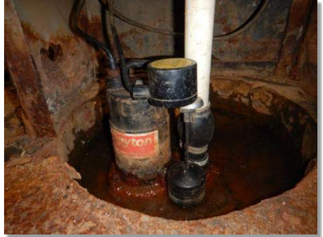
Photo 3-70. Moderate corrosion at sump
