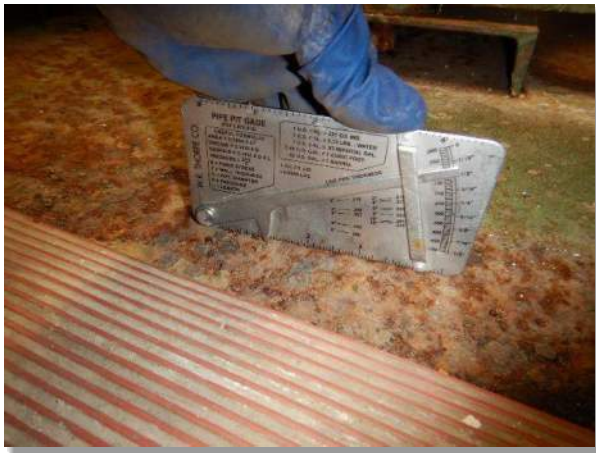
Photo 3-13. Moderate corrosion at floor plate, pits up to 0.07-in
