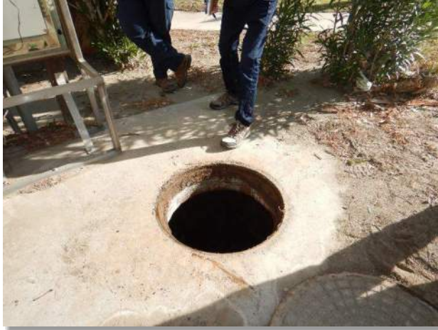
Photo 3-15. Wet well access
