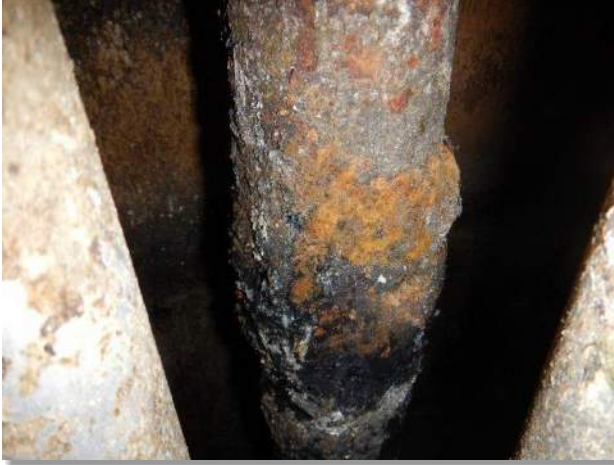
Photo 3-91. Severe corrosion at Pump 1 discharge piping, close-up
