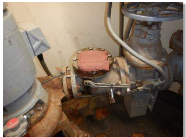
Photo 3-62. Pump No. 1 discharge piping & valves
