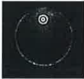
RELATIVELY CLEAN SIPHON
