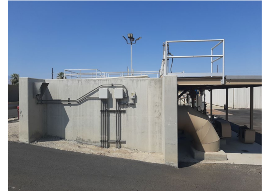
Existing Aerated Grit System – to be decommissioned
