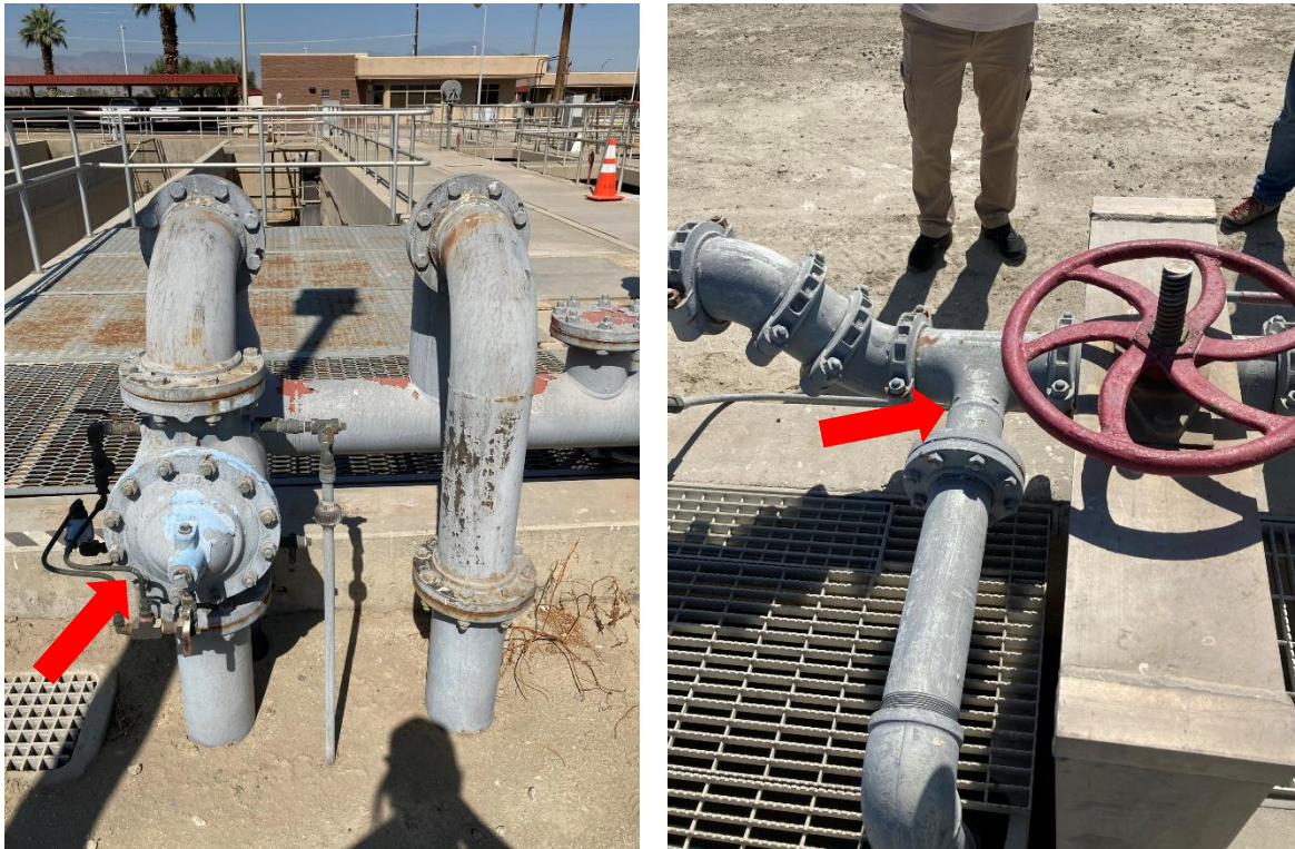
Figure 2: Project Start Location – 6” Regulating Valve (left) and Valve to be added to Lateral (right)
