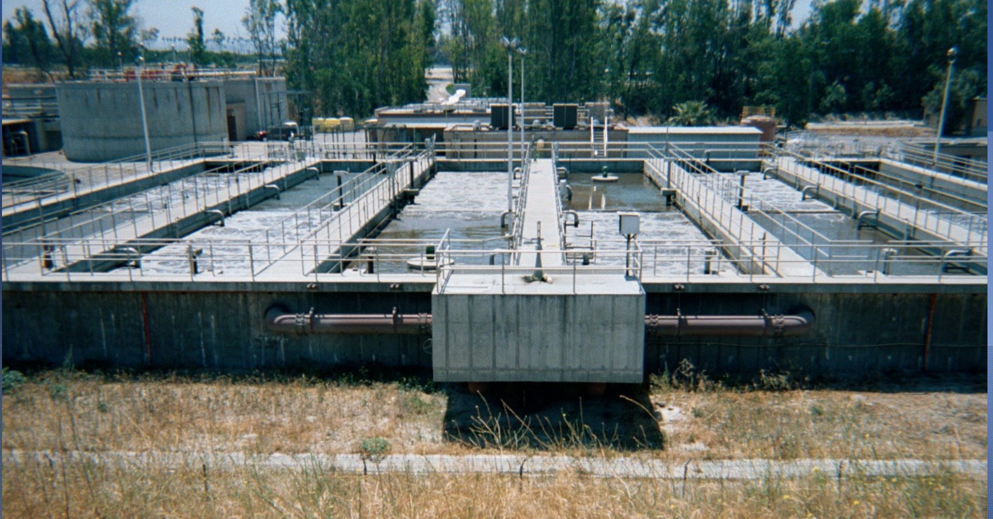
City of Redlands CA WWTP in Step-Feed Mode
