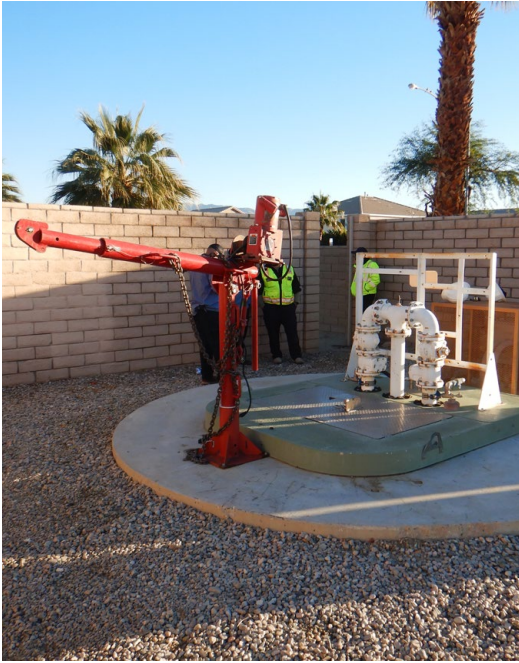
As part of Harris' Program and Design Management Collection System Infrastructure Project, we managed the completion of Calhoun Lift Station condition assessment.
