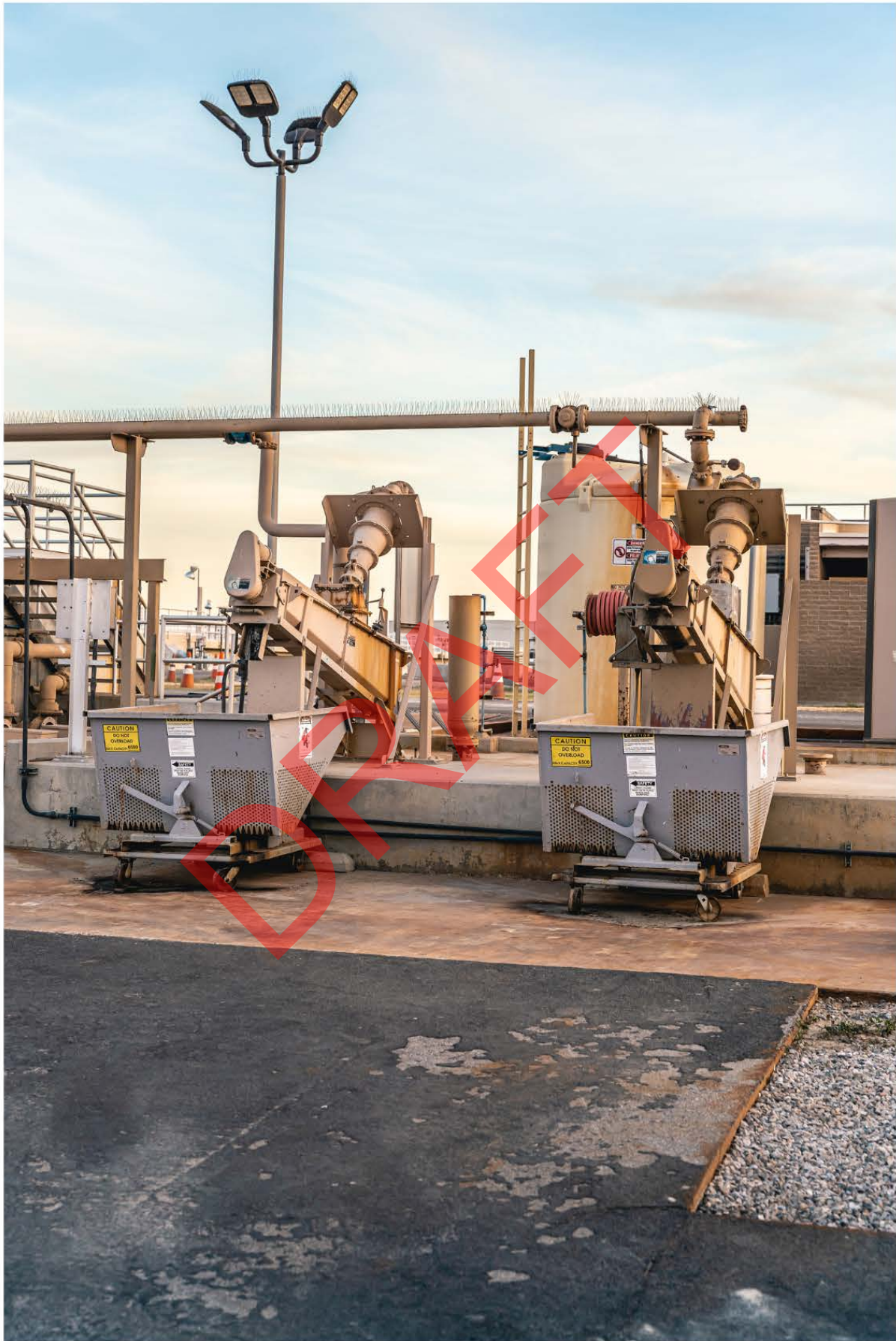
Wastewater Facility Grit Hoppers
