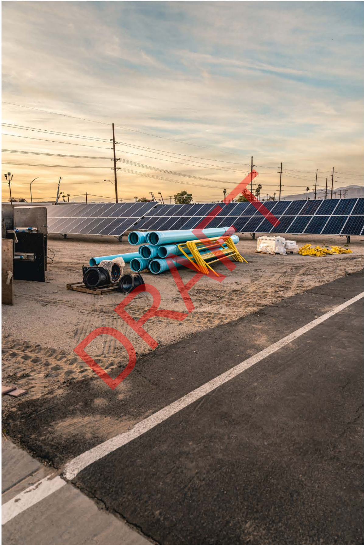
Wastewater Facility Recycled Water Project Sewer Piping
