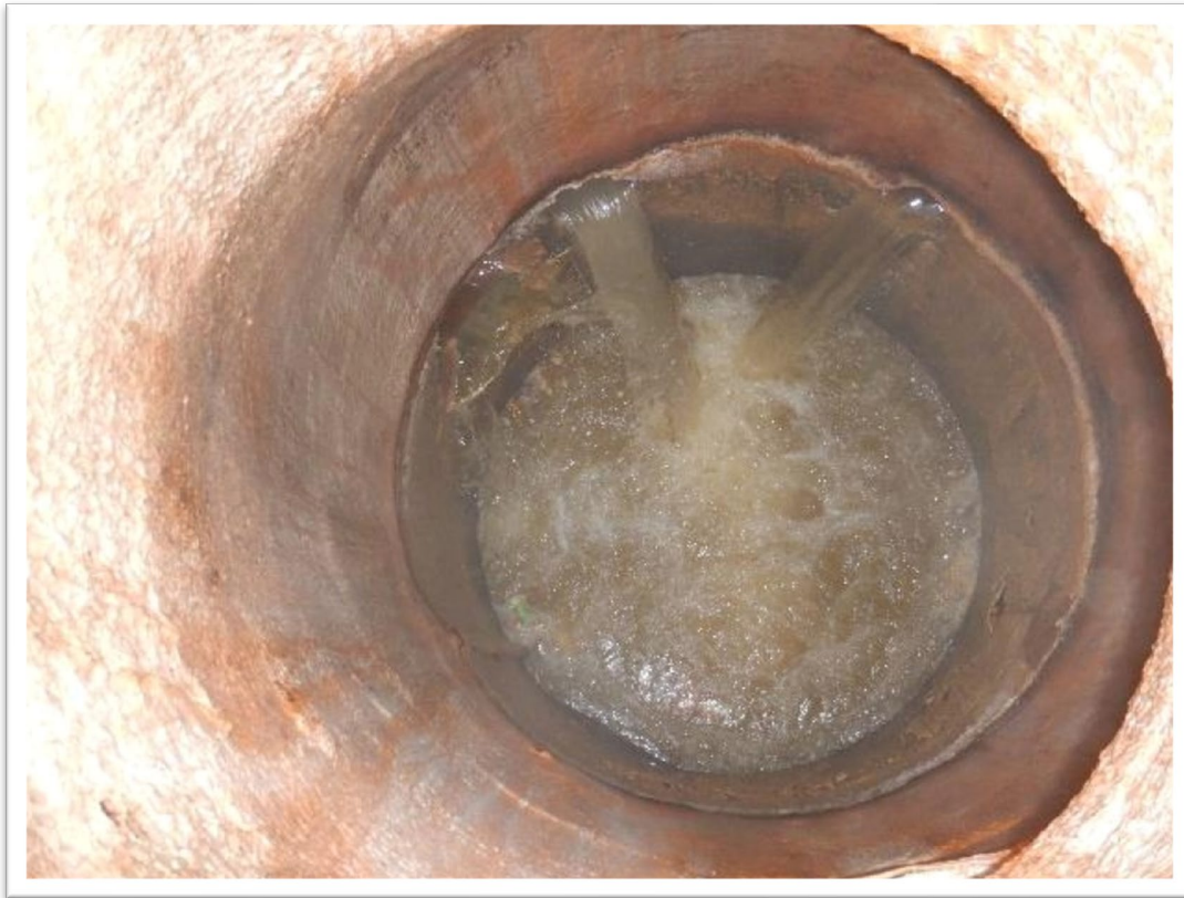
Photo #1: Carver Lift Station Wet Well
