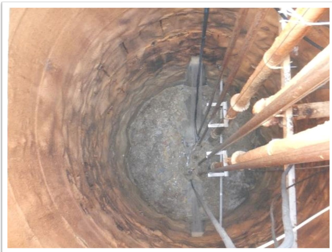
Photo #2: Calhoun Lift Station Wet Well
