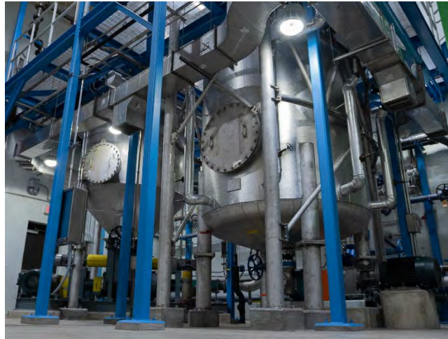
Figure 3-2 Lystek LY10 Module installed with dewatered biosolids storage tank (left) and Lystek THP Reactor (right)
