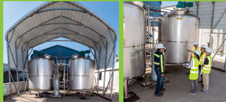
Refeeding of the Lystek-processed material into anaerobic digesters results in higher volatile solids breakdown, higher gas yields, and reduced biosolids volumes.
