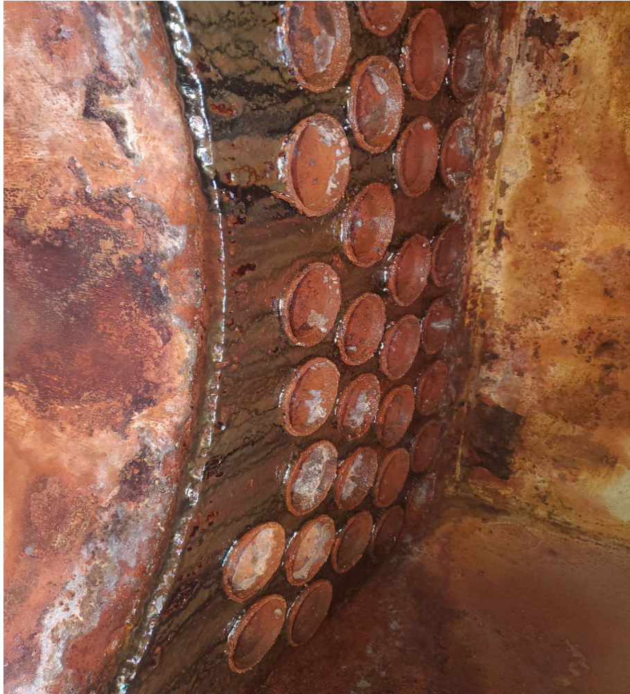
Damaged Heat Transfer Tubes
