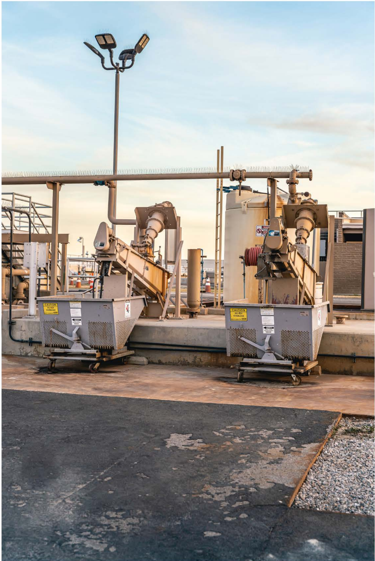
Wastewater Facility Grit Hoppers
