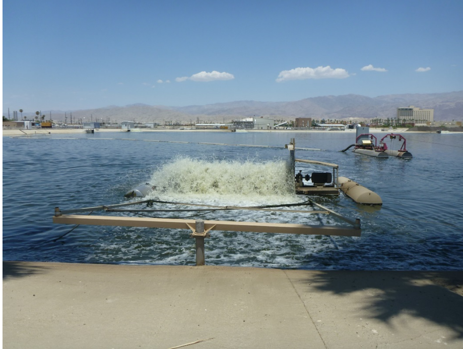
Figure 3-8 Pond 2 and Surface Aerator
