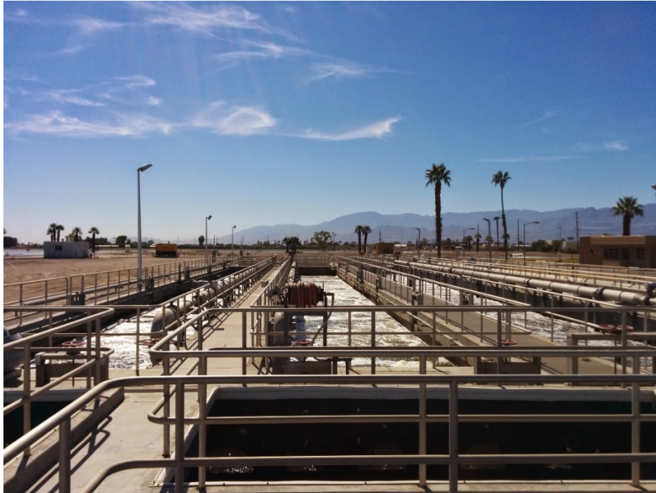
Figure 3-5 Activated Sludge Selectors and Aeration Basins
