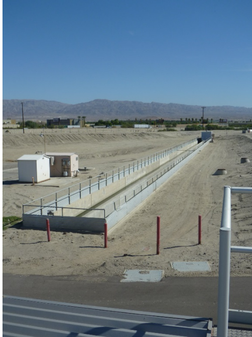
Figure 3-11 Chlorine Contact Tank 2
