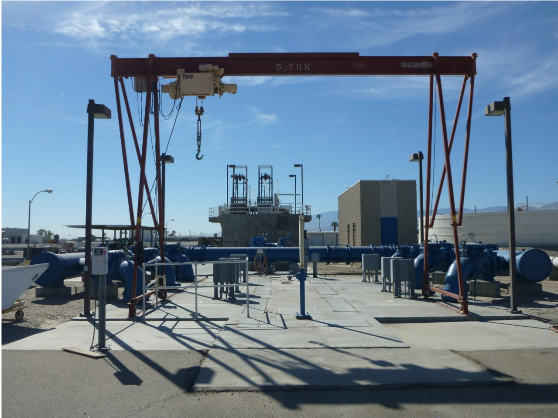
Figure 3-2 Influent Pump Station
