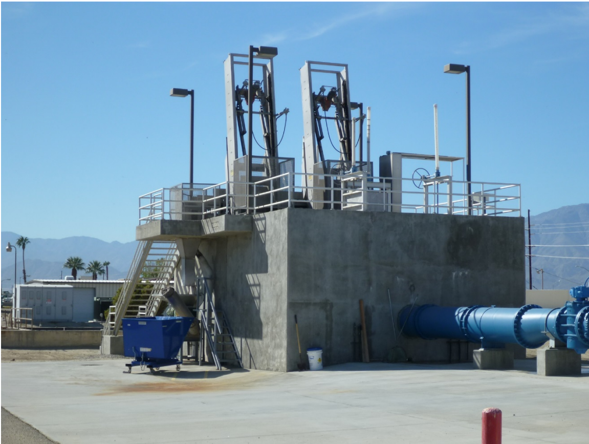
Figure 3-3 Screening Facility (Bar Screens)
