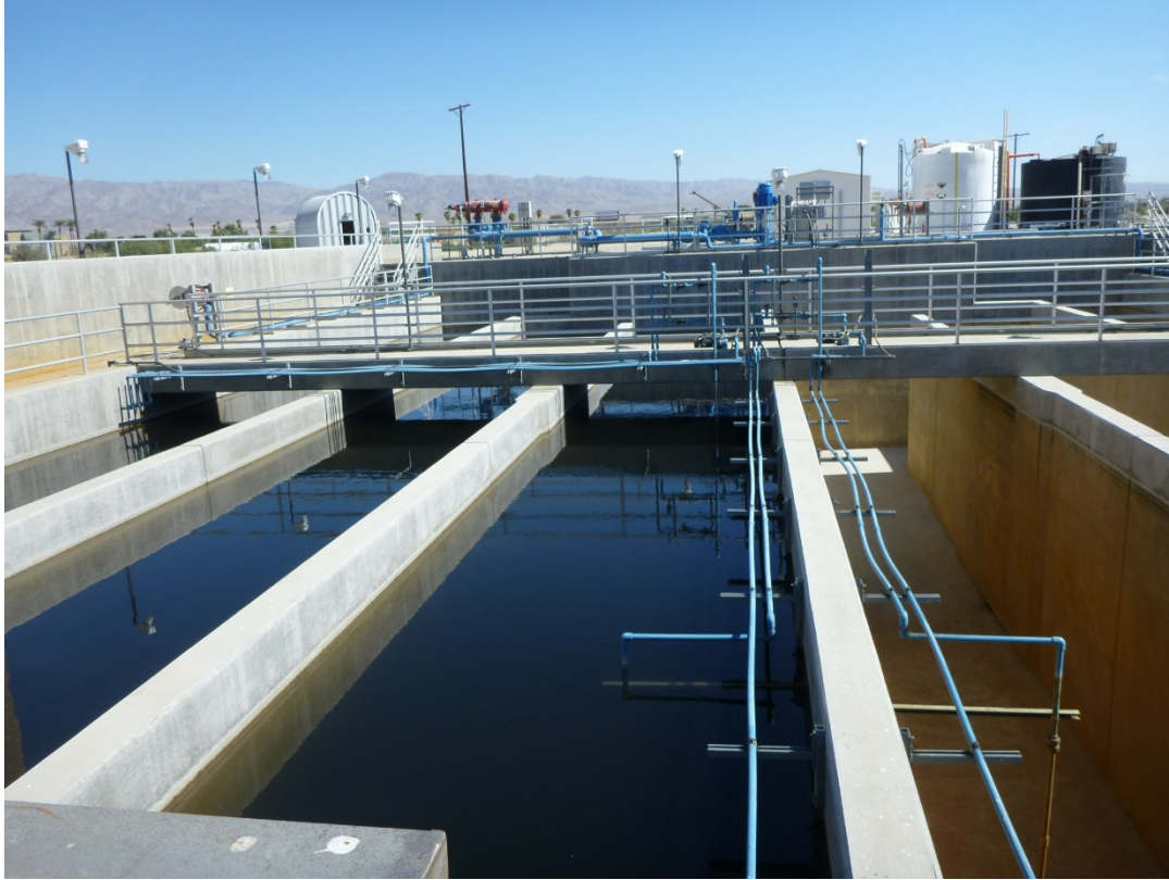
Figure 3-10 Chlorine Contact Tank 3
